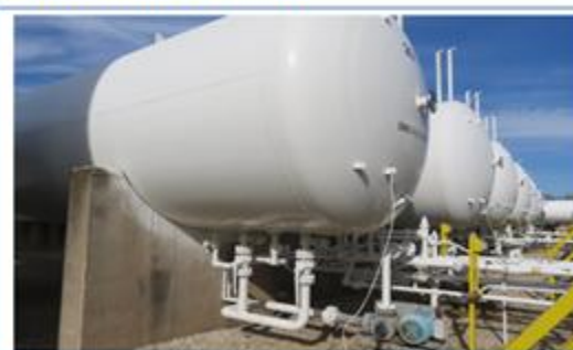
DME Storage Tank
